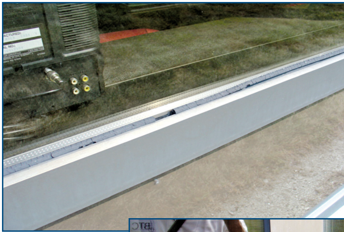
Photo 1 - Cracking of glazing gaskets in a curtain wall system.
