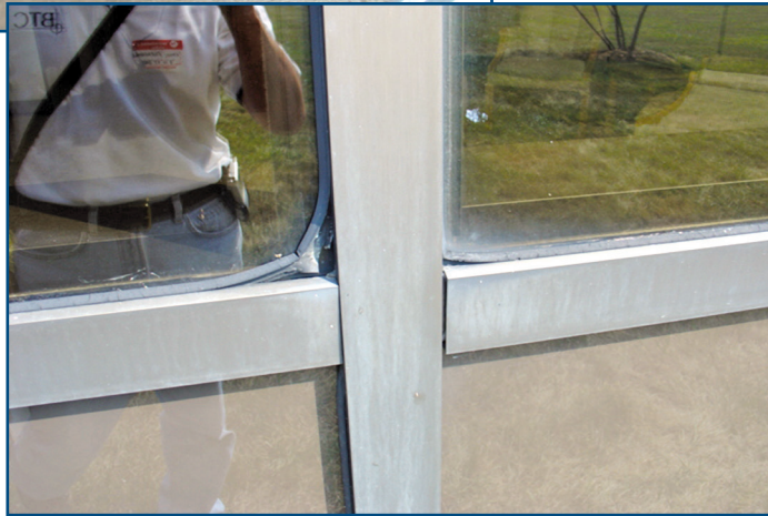
Photo 2 - Shrinkage of glazing gaskets.
