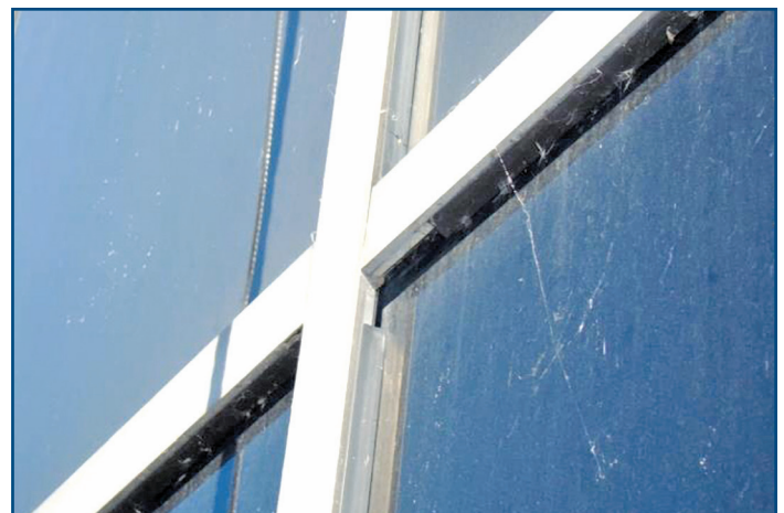
Photo 3 - Extruded glazing gasket shrinkage.
